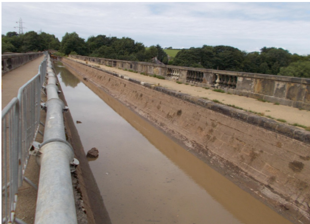
The dished stone lining of the aqueduct is revealed by the draining of the water. The pipe carries the water flow from the north past the stoppage.
