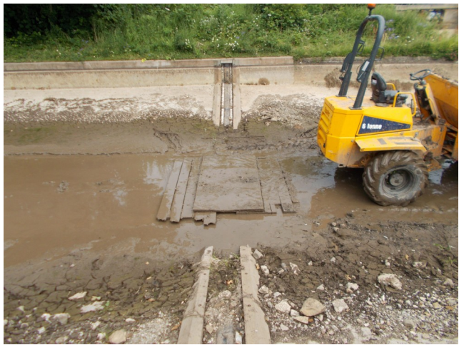
The seal where the puddle canal to the right meets the stonework of the aqueduct. The planks protect the seal from the machines which ran along the bed of the canal to carry out the maintenance and repair works
