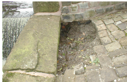
Damage continues after repairs
